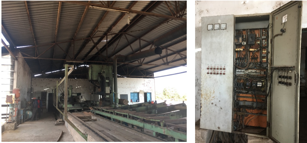
Figure 4: General aspect of wood processing factory (left) and electrical cabinet (right)
