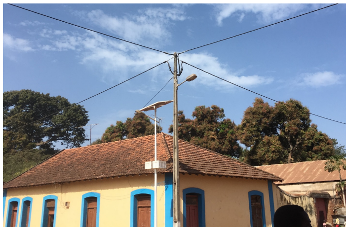
Figure 2: Solar street light (left) and grid-connected one (right) in the administrative district of Bissorã
