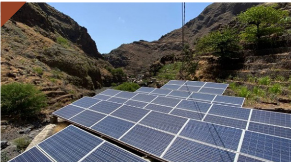
CABO VERDE (SANTO ANTAO) Refurbishment of Ribeira Alta's Hybrid Power System
