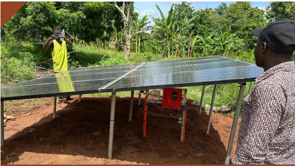
BENIN - Solar-Powered Irrigation System (SPIS) installed at the Adja-Ouère Agricultural Technical High School
